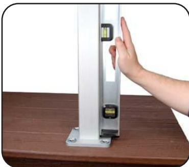
Step 4: Ensure post is plumb, adjust as needed. Tighten fasteners and ensure proper engagement into blocking.
